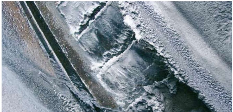
Hard scale deposit behind turbine inlet nozzle
