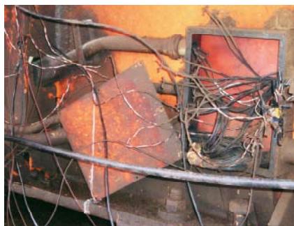
Old wiring around junction boxes
