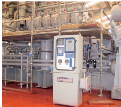
Altronic Air/Fuel Ration Control Panel with vibration monitor and CPU-95 display.
