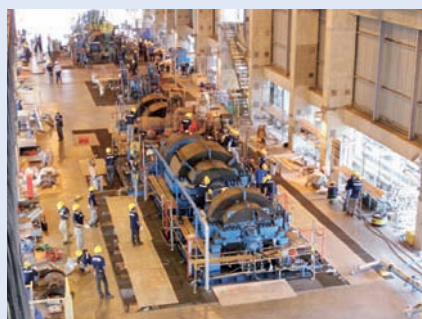
9 machines all awaiting overhaul.
