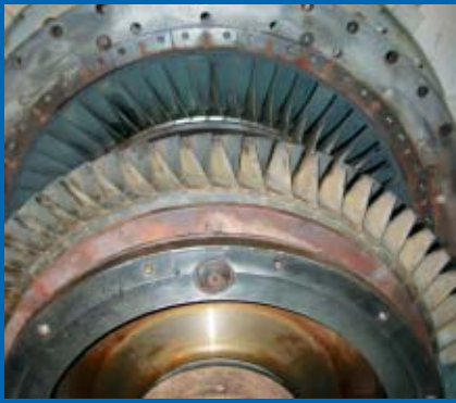
1st stage buckets to 2nd stage buckets.
