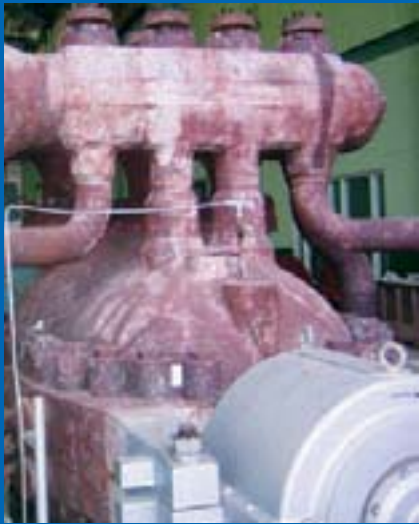
Steam Turbine without insulation
