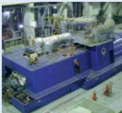
Steam turbine back in operation after overhaul.
