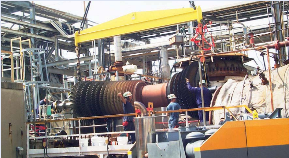
50 MW Swiss-designed gas turbine in one of the largest chemical plants in the US.
