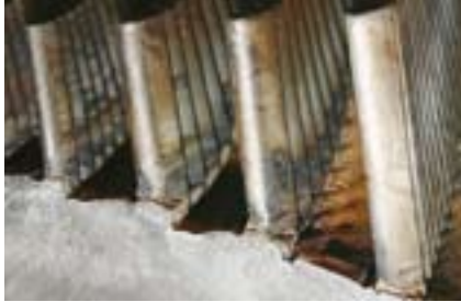
Stationary blade erosion.
